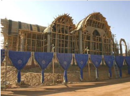
Figure 12 New Church at Anba Hidra, West Bank, Aswan, under construction (Howard Middleton-Jones 2010)
